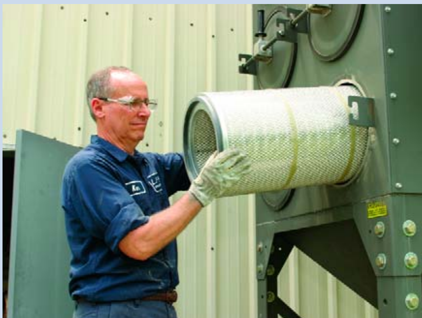
When the pressure drop rises 1 to 2 inches water gauge above the normal static pressure, it's probably time to change your filters.
